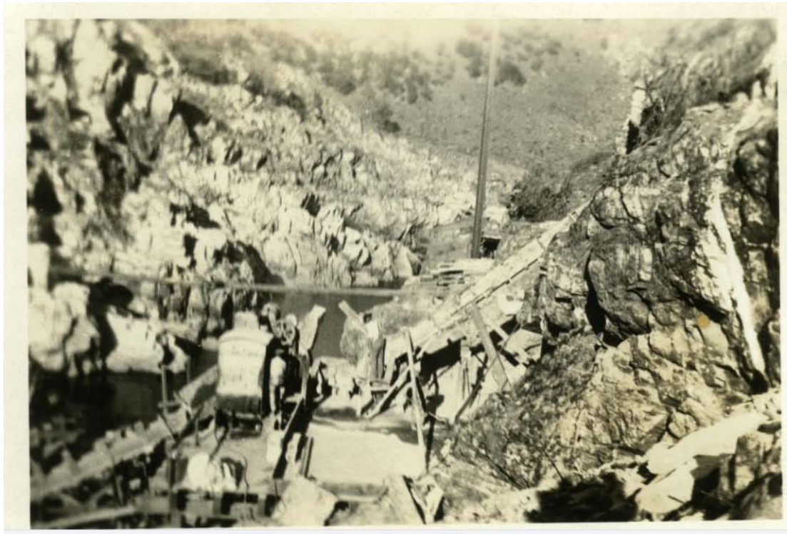
Figure 12.1 Early construction on Old Don Pedro Dam circa 1922. One construction worker appears to build one of the wooden chutes used to convey concrete. Another man is visible by the large machine which is probably a cement mixer. The Old Don Pedro Dam was designed and constructed on the Tuolumne River, northeast of Turlock, California. The project began in 1921 and was completed in 1923. Almost 300,000 cubic yards of concrete was used to build the dam and spillway. From http://www.calisphere.universityofcalifornia.edu/ . California State University, Stanislaus. University Library. Special Collections
